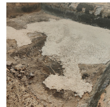
Repair example: Ingot mould bottom
