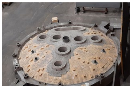
Also available in slow setting version (2 hrs max.) e.g.: heart of roof blocking
