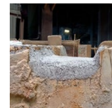
Repair example: Tundish spout
